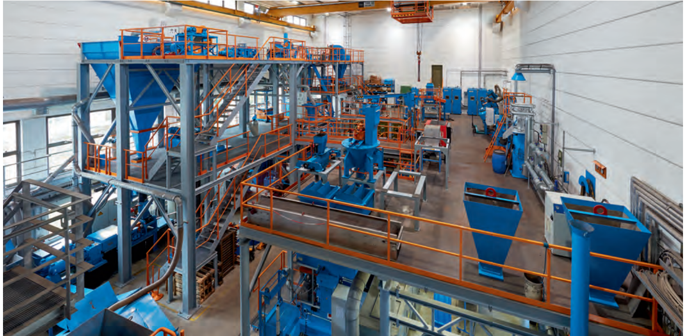
Overview of pilot plant
